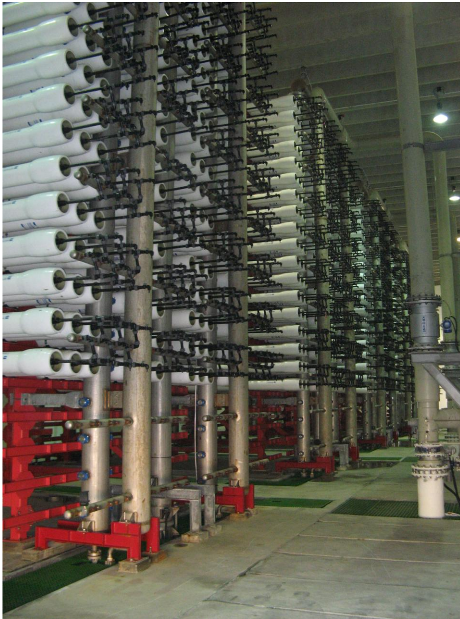
Figure 5: Palmachim desalination plant
