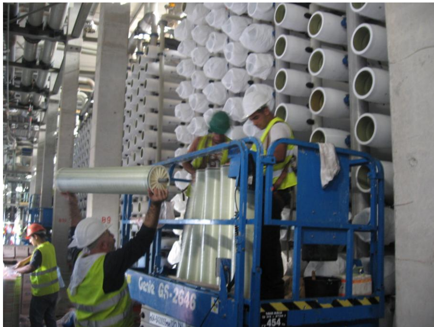
Figure 6: Hadera desalination plant
